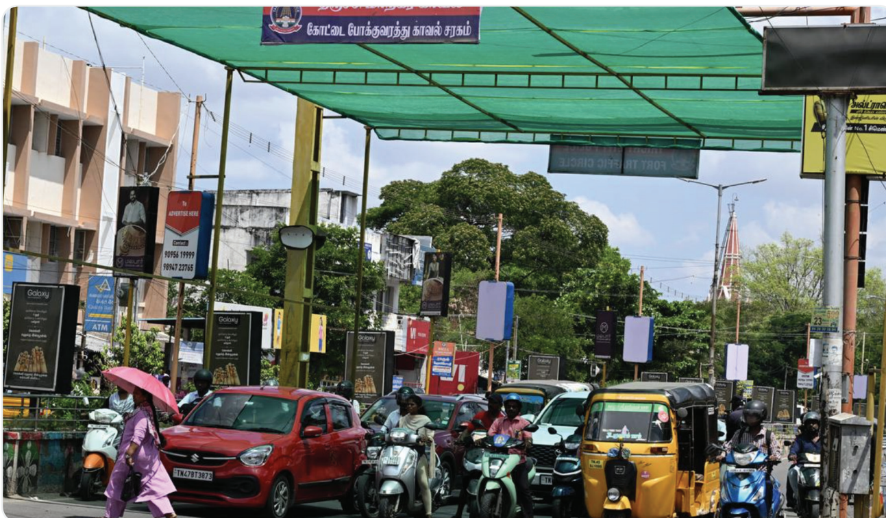
Figure 29: Canopy installed at the traffic signal 63 / junction at Puthur Road in Tiruchi, Tamil Nadu
